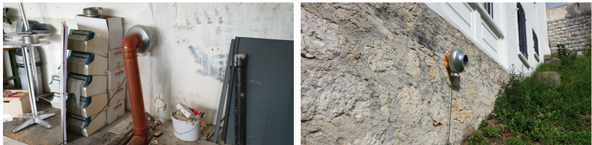
Picture 1: Installation of one sump under the closed office (left) and another sump under the stairway (right)
